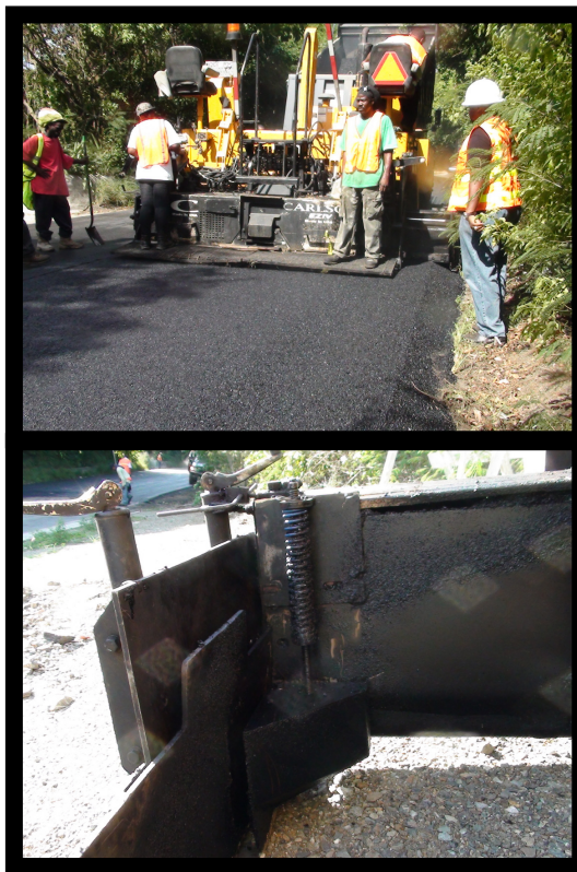
Pictures from the Test Site of the Safety Edge on Route 70 in Saint Croix, US Virgin Islands.
